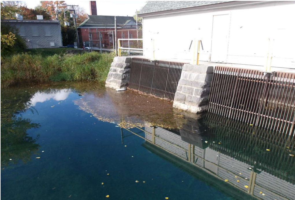
Photo 6 Dam ID# 073-0355 Skaneateles Lake Dam 10/23/2023 Service spillway obscured by vegetation at the left end of the dam.
