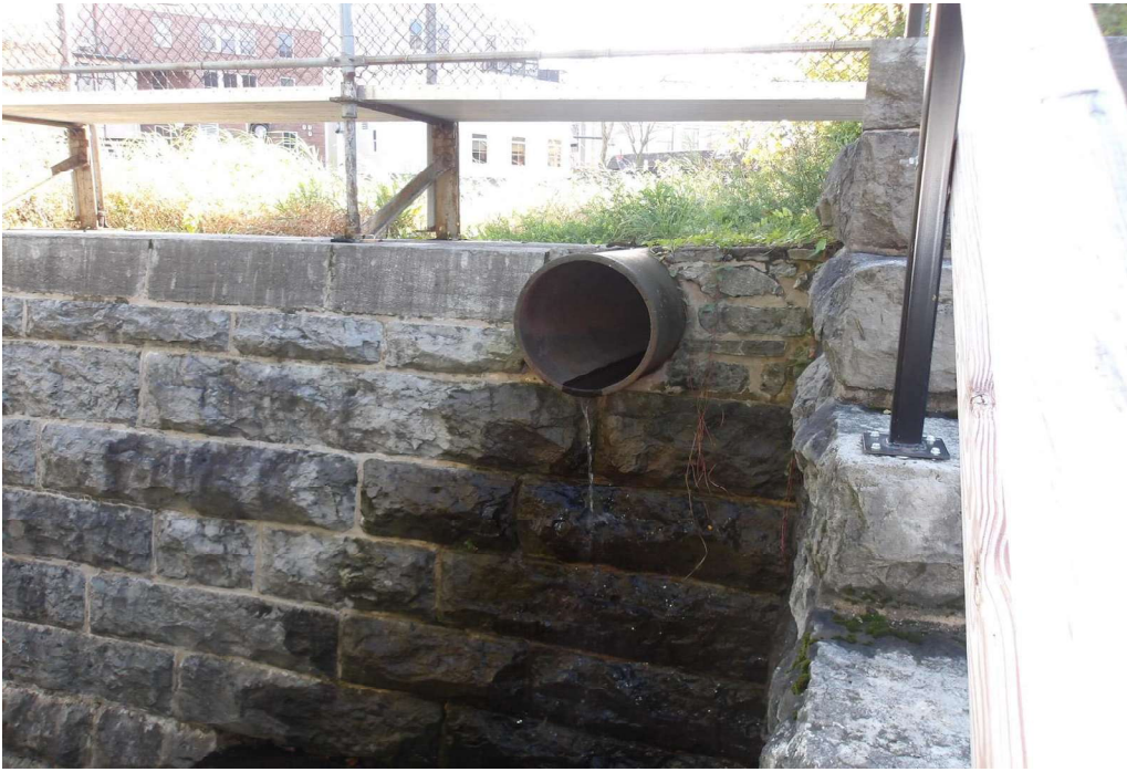
Photo 7 Dam ID# 073-0355 Skaneateles Lake Dam 10/23/2023 Left downstream groin with pipe observed leaking.
