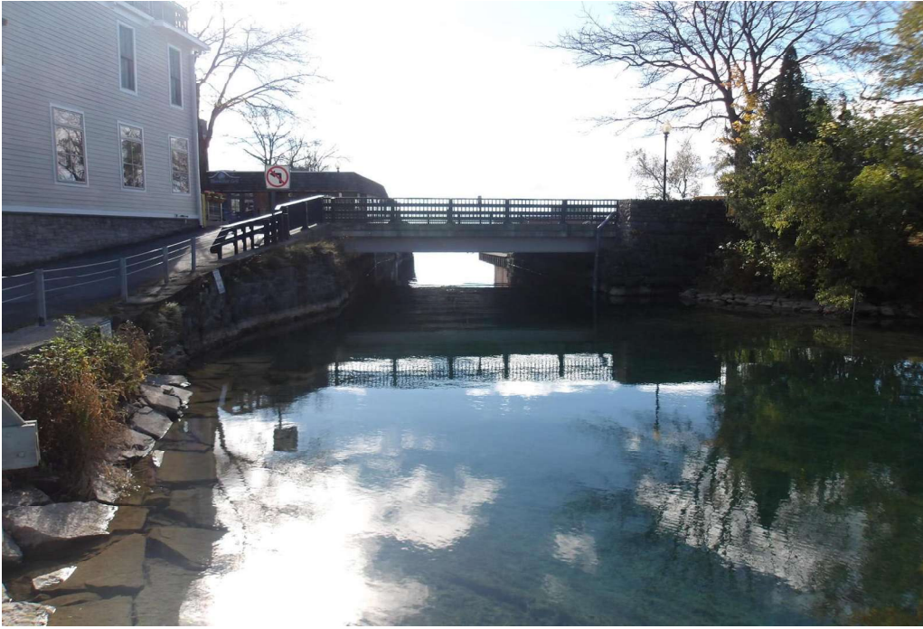
Photo 9 Dam ID# 073-0355 Skaneateles Lake Dam 10/23/2023 Approach channel to the dam, looking upstream.
