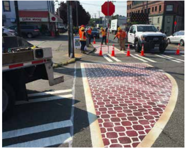
An example of a painted curb extension in Seattle, Washington. (Photo: Seattle Department of Transportation)
